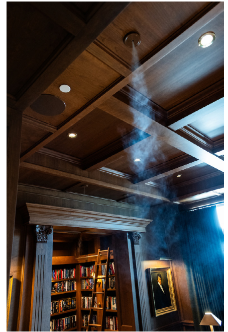
Marko Residence Library with custom painted MN spray heads
