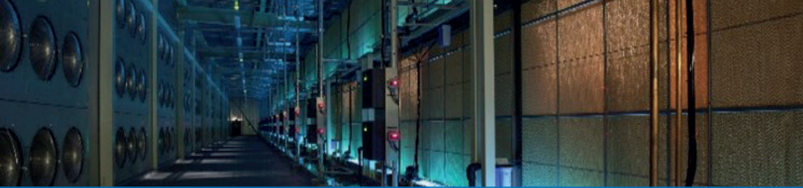
Image: A double height ME Series humidification system cools a data center in Sweden.
